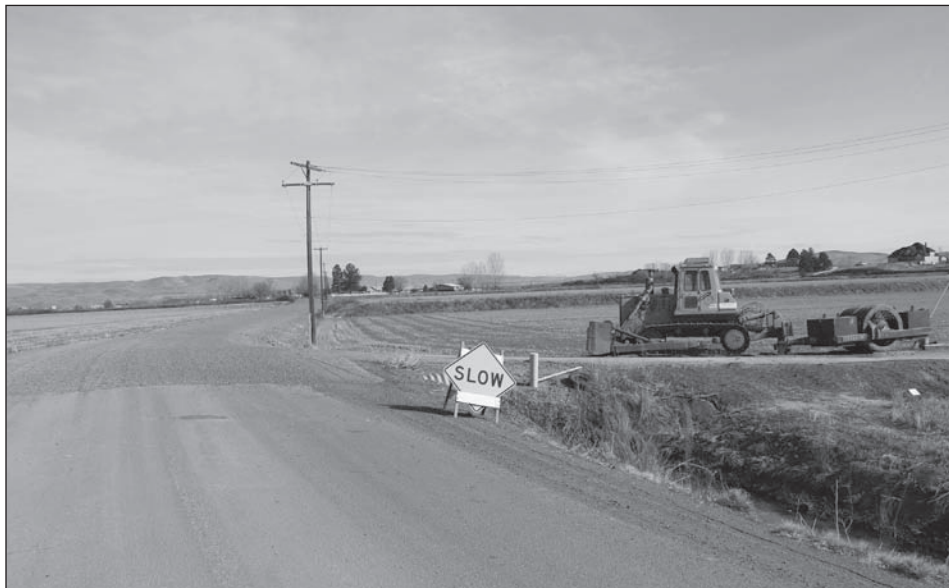
The Washington County Road and Bridge Department repaired and upgraded three spots on Cove Road, including rebuilding the section above, and will pave the gravel portions with three inches of asphalt when it warms up. The county also plans to pave a short portion of Mann Creek Road where a pipe was installed and a patched-up part of Old Highway near Midvale. Photo by Steve Lyon
